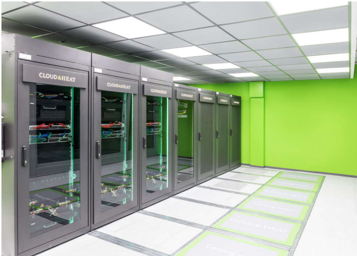
Illustration 2: Cloud&Heat server room in the Eurotheum, Frankfurt/Main
